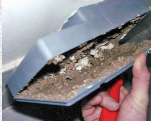
Above ground station with termite activity.
