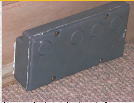
Above ground station placed on damaged wall.
